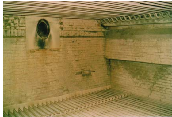
Fig. 2 A view of the refractory wall around the wave entry port above economizer tube package after 15 months of continuous operation of DSB.
